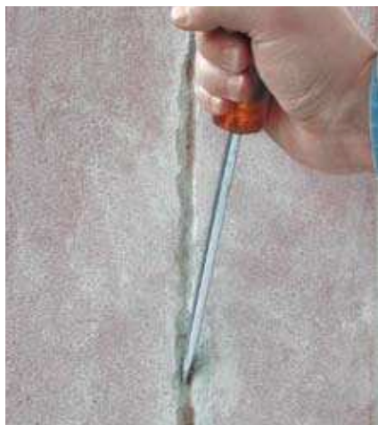
(1) Expanding the crack
