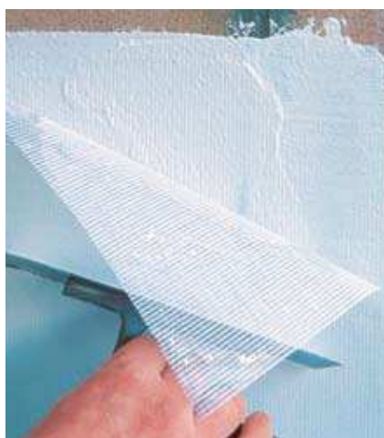
(5) Application of RIALTO FIBRELAST and leveling treatment with second coat of RIALTO RASELAST
